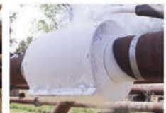
Diagonal frostline indicates ice plug is forming. When freezing is complete, repairs can be made.
